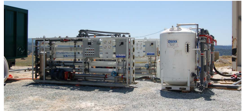
Front view of RO unit and multimedia prefilter
