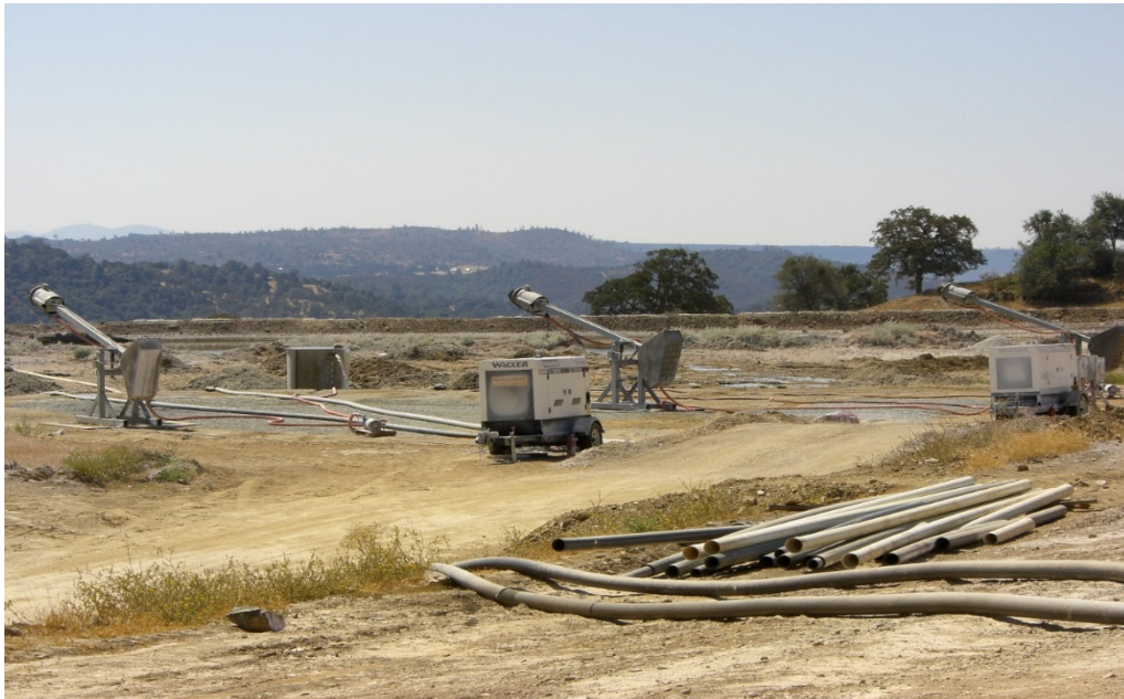
Three spray evaporators, not operating yet
