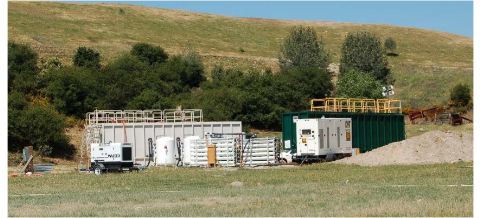
Example: Two frac tanks, multimedia prefilters, two RO skids, generator
