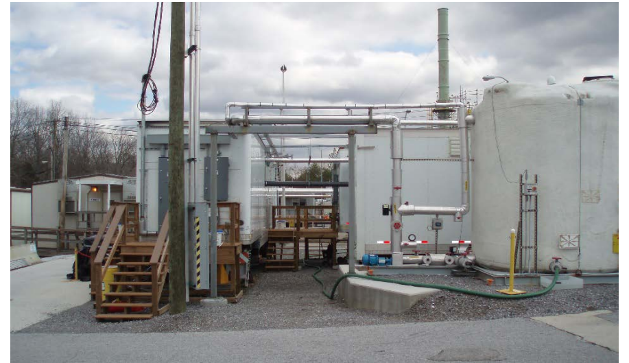
Two of the trailers installed at the facility
